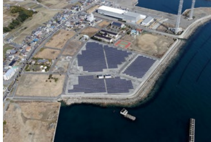
PV systems for a 2MWp solar plant on Awaji Island in Japan
