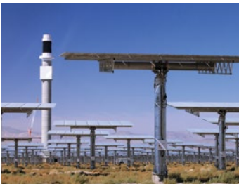
Solar tracking systems for a power plant in the U.S.A.
