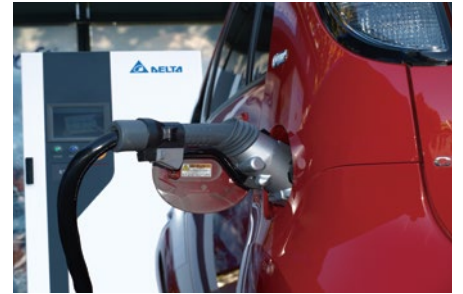
EV charging solutions for a charging network in Norway
