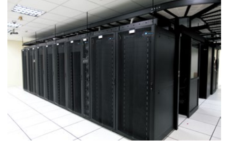
InfraSuite datacenter infrastructure solutions for National United University in Taiwan
