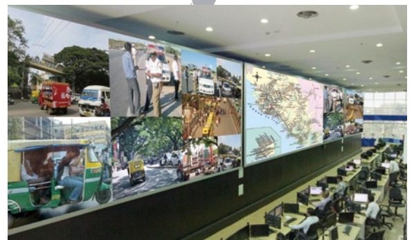
LED-based DLP Video walls for the first traffic management center in Bangalore, India
